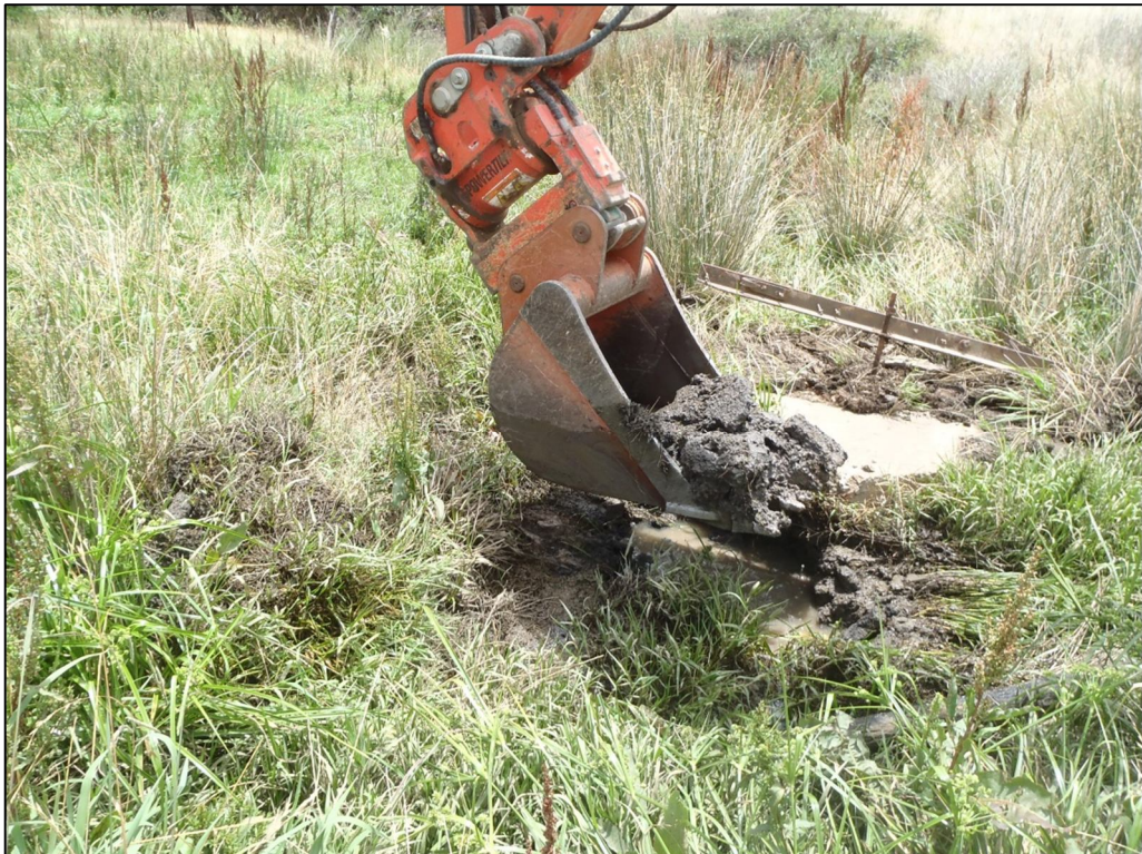
Plate 20 – Concrete and asphalt observed dumped in Barnes Gulley in the northeast portion of the site.
